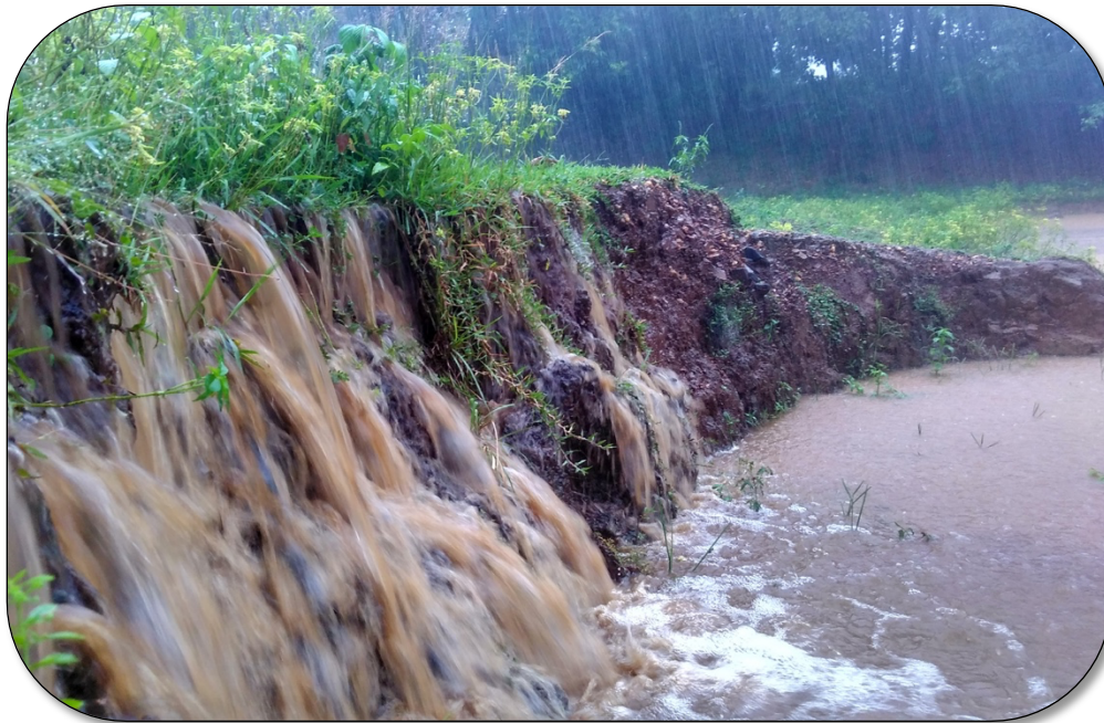
Image 22 This private pond that has experienced catastrophic bank collapse due to poor buffer zone design and heavy ground water flow.
